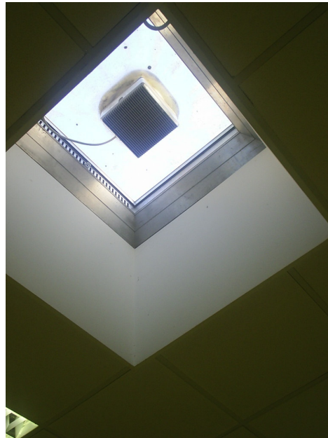
Figure 3.2 Ventilation fans in ceiling
