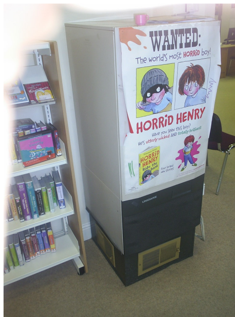
Figure 3.1 Storage heating unit
